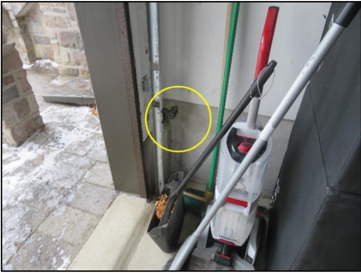
Sensors poorly located
