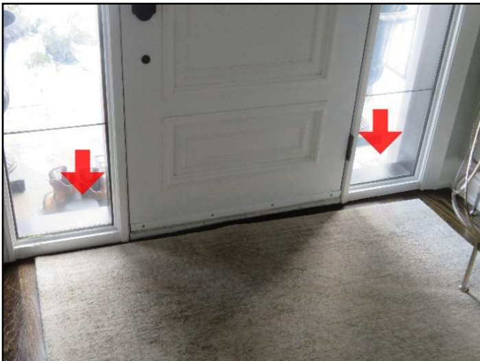
Lost seal on double glazing
