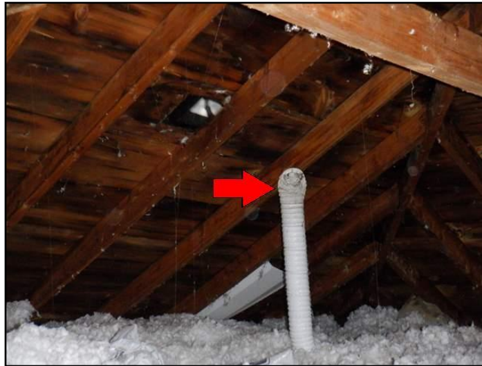
Not vented to exterior. Not insulated
