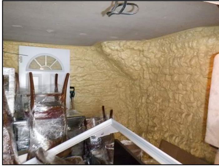
Exposed combustible insulation
