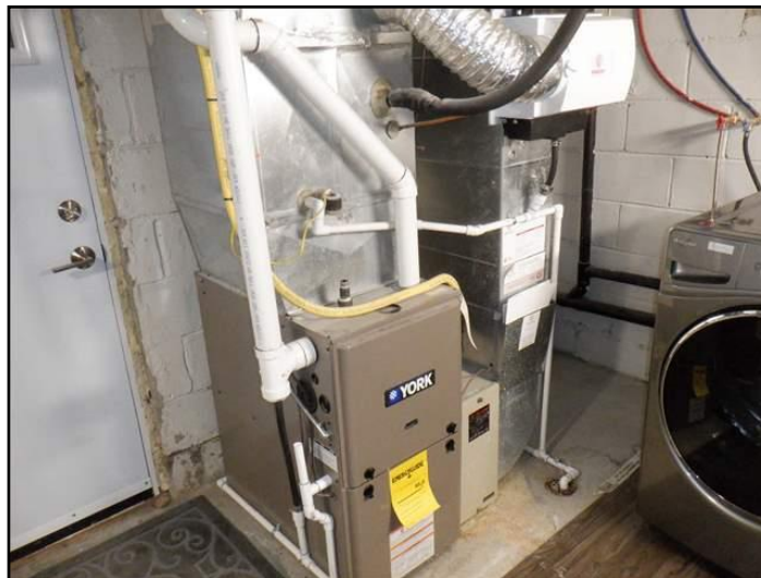
Furnace (high efficiency) 15 to 20 years
