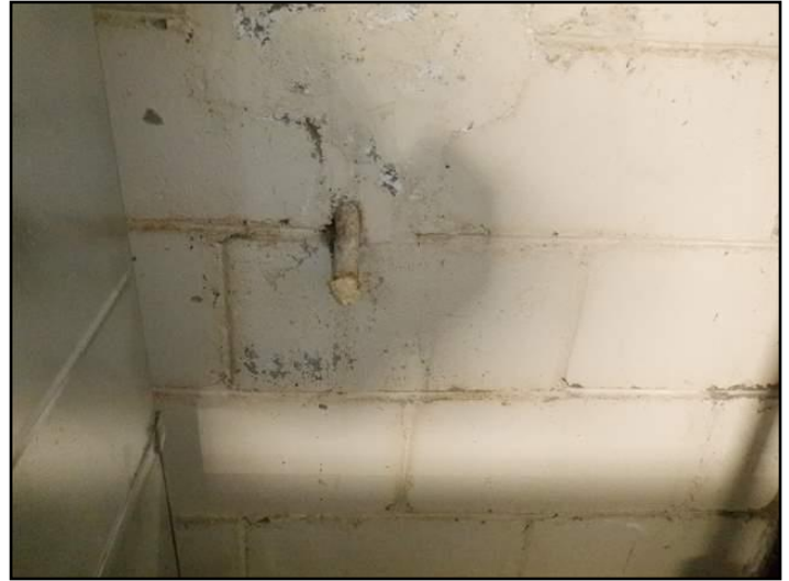
Unknown abandoned pipe
