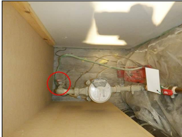
Main water shut-off valve
