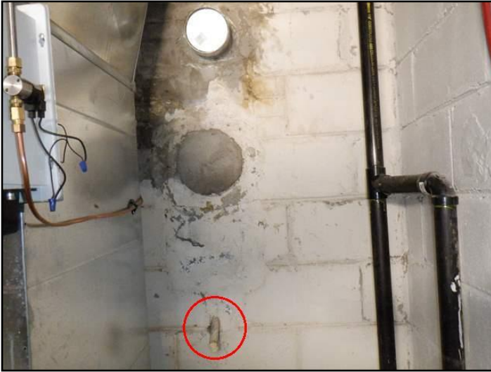
Unknown abandoned pipe
