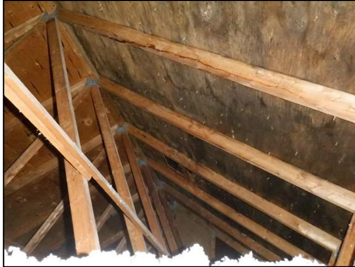
Mould in attic
