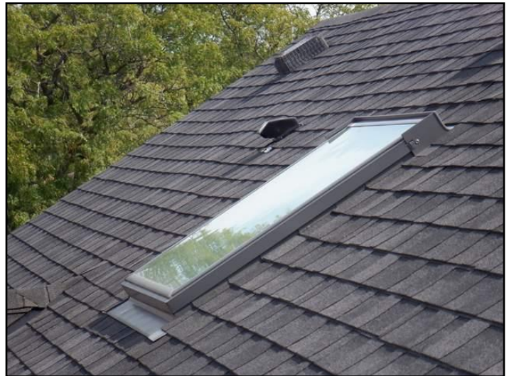
Curb - low, missing
