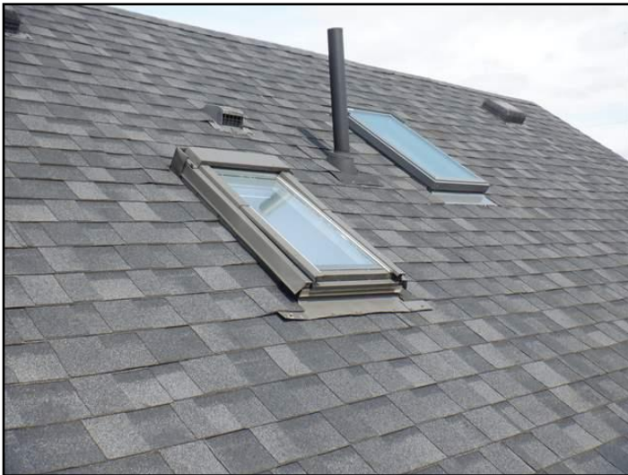
Curb - low, missing
