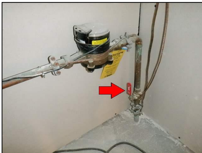
Main water shut-off valve
