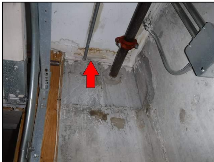
Water stains beside vehicle door...
