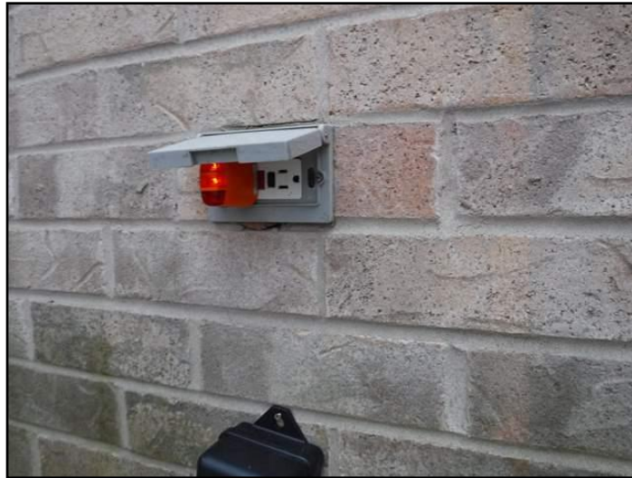
Test faulty on GFCI/GFI (Ground Fault...
