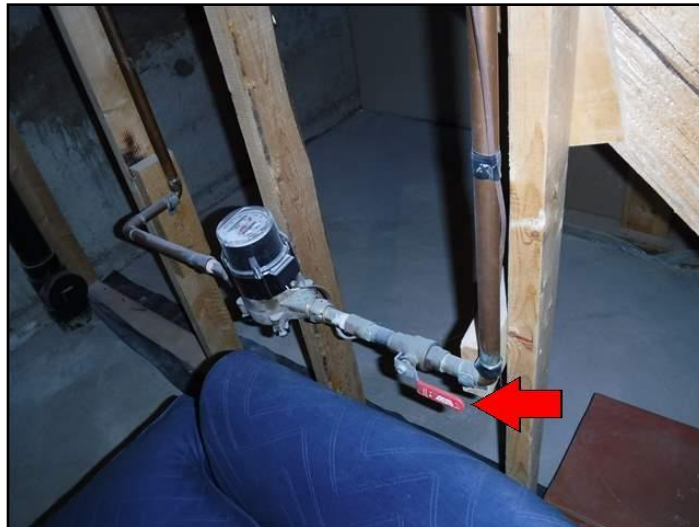
Main water shut-off valve
