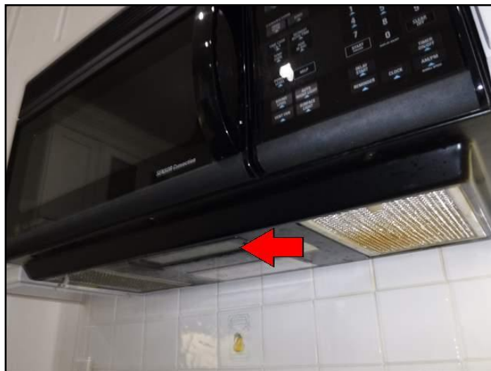
Work light inoperative
