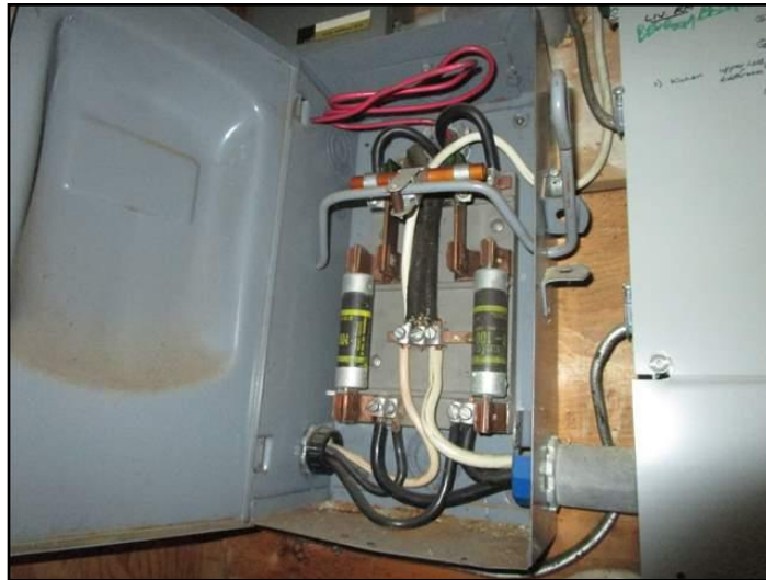
Fuses - basement (panel cover opened)
