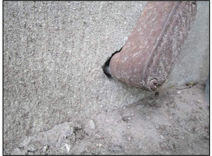
Caulking missing or deteriorated
