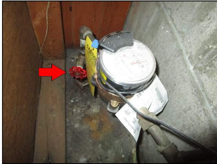
Main water shut-off valve
