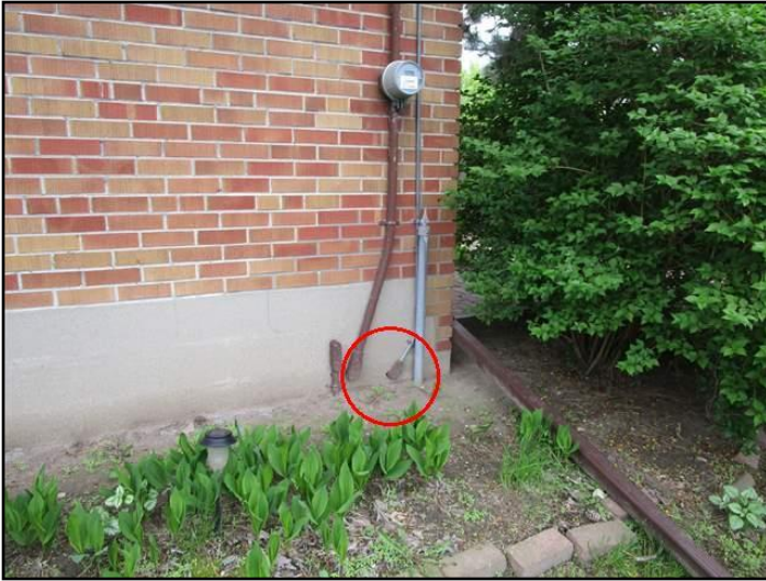
Caulking missing or deteriorated
