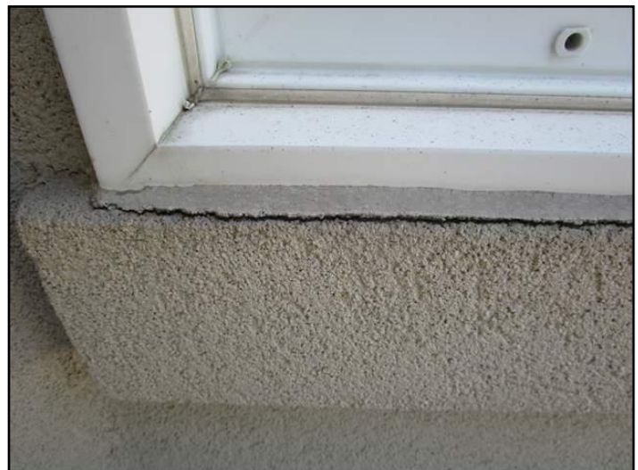
Caulking missing, loose or deteriorated
