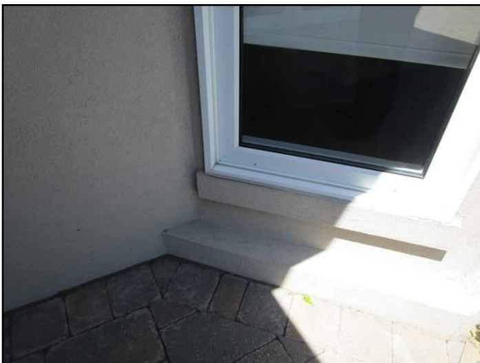
Caulking missing, loose or deteriorated
