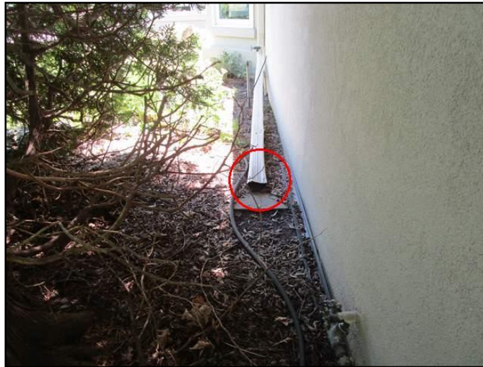
Discharge too close to building
