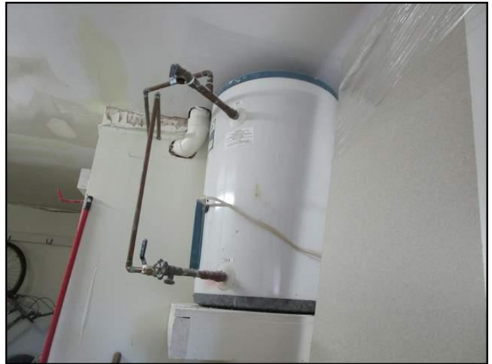
Discharge tube missing
