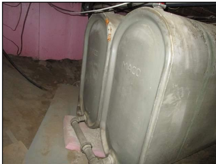
Abandoned oil tanks
