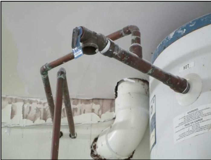
Discharge tube missing
