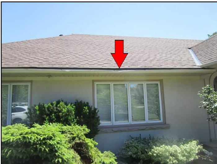
Improper slope, ponding
