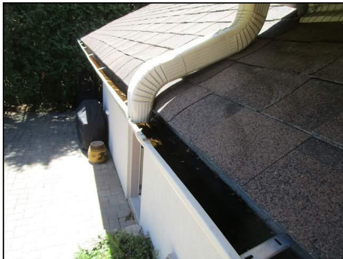
Improper slope, ponding
