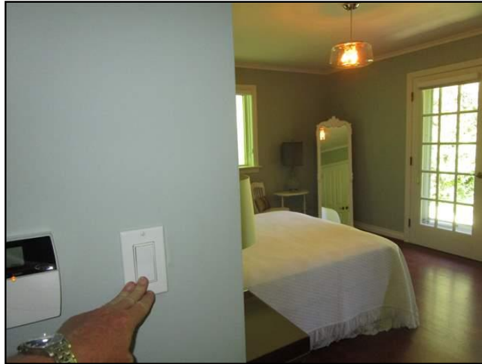
Light switch inoperative or not found
