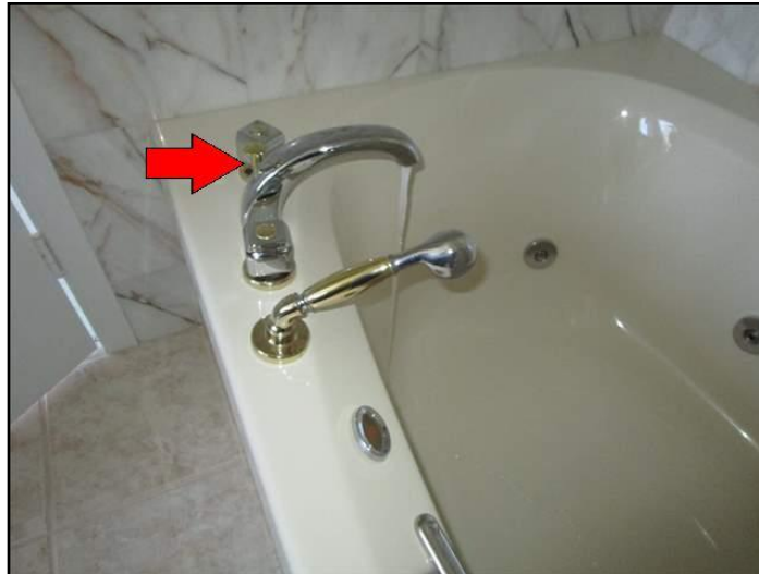
Diverter stiff/difficult to operate
