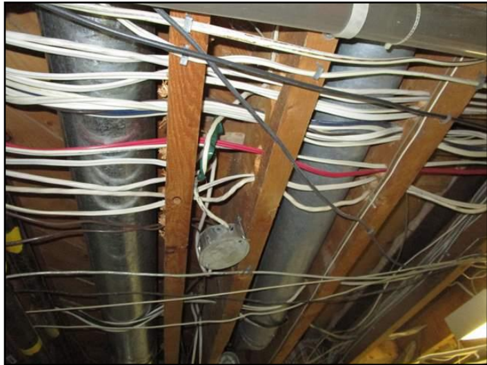
Too close to ducts
