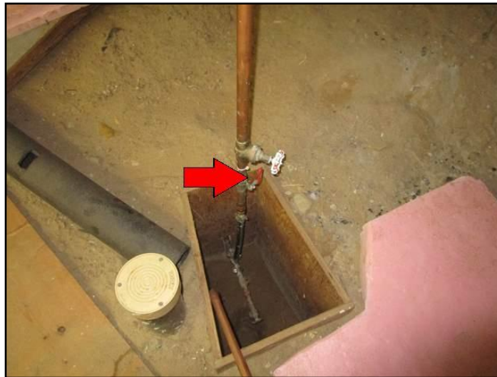
Main wate shut-off valve
