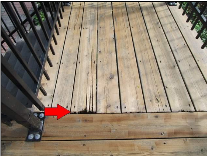
Weathered - Rot noted at various plank ends
