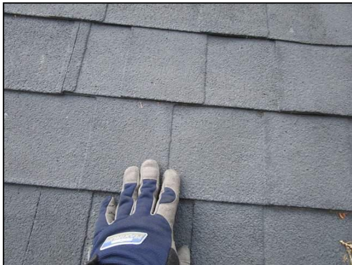
The shingles appear to have been coated...
