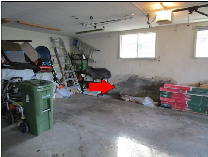
Prior repairs noted to walls...
