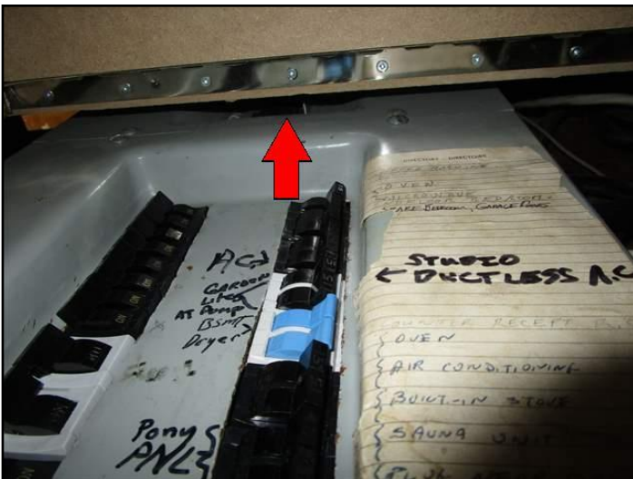
Poor access to main disconnect
