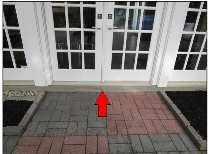
Threshold - too low
