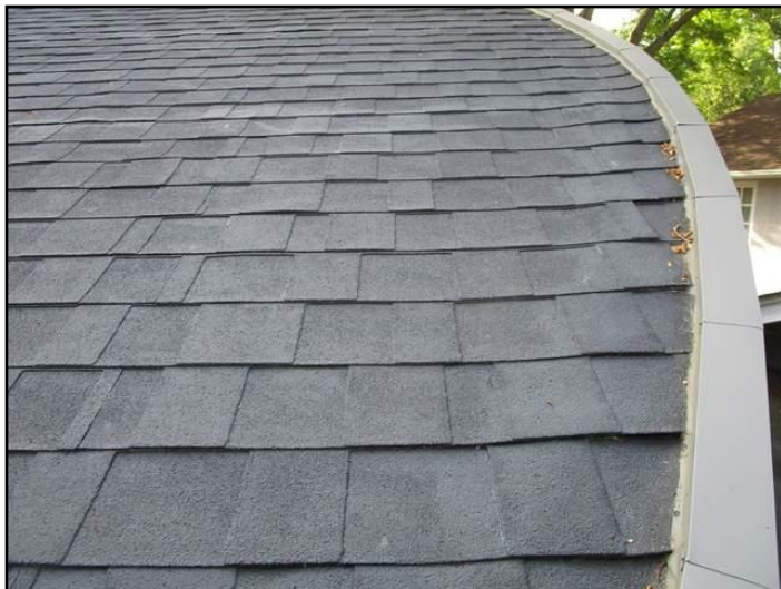
The shingles appear to have been coated...
