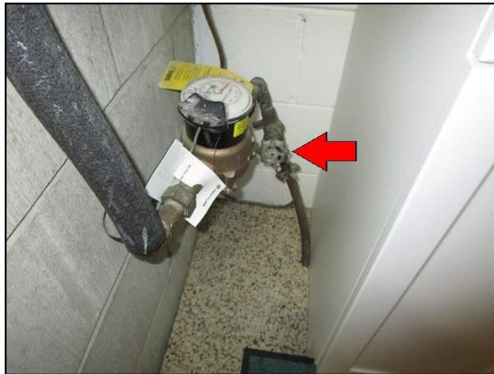
Main water shut-off valve
