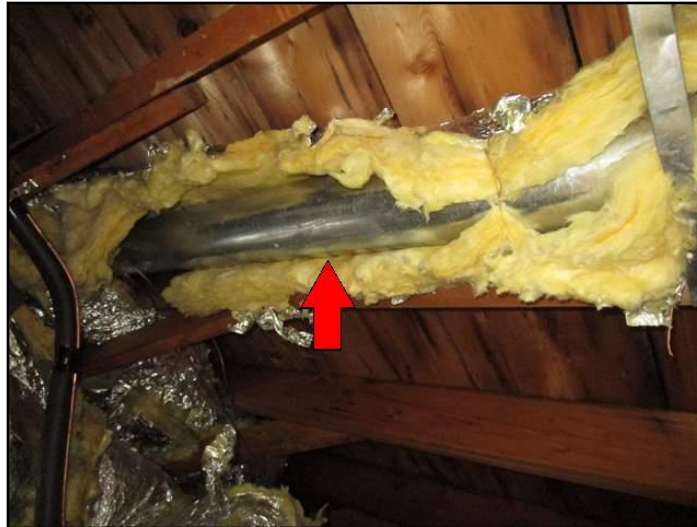
Not insulated in unconditioned space
