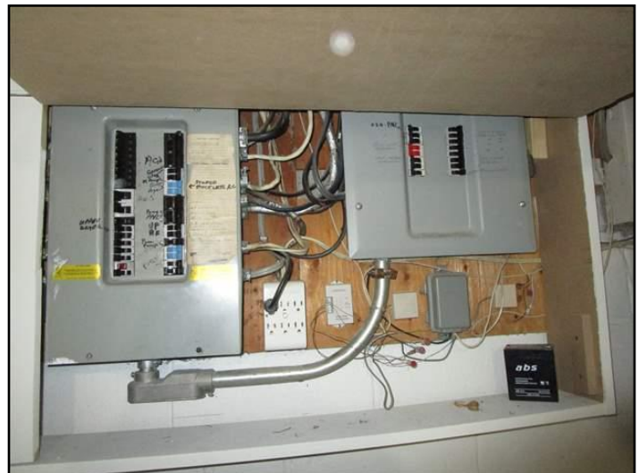
Panel covers not removed...
