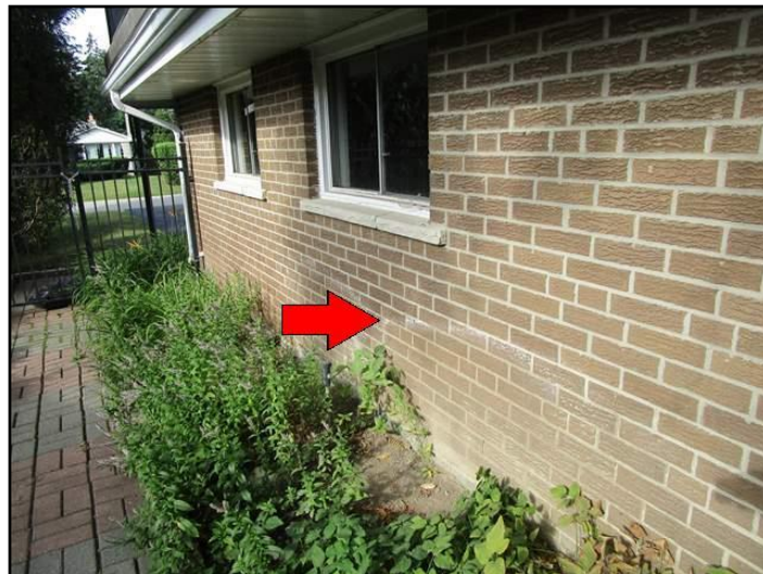
White stains show water has entered brick...
