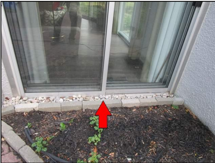
Threshold - too low
